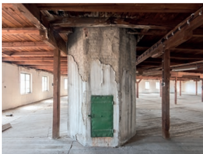
Figure 4: Roof part of the pedestal on the fourth floor of no. 1148 with a closed door (probably coupled with some type of grate in the chimney flue).
