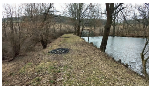
The Bavorovský Stream, The Bavorov Reservoir – Reservoir reconstruction and de-watering reservoir, condition before repair (Author: Bušek Jan)
