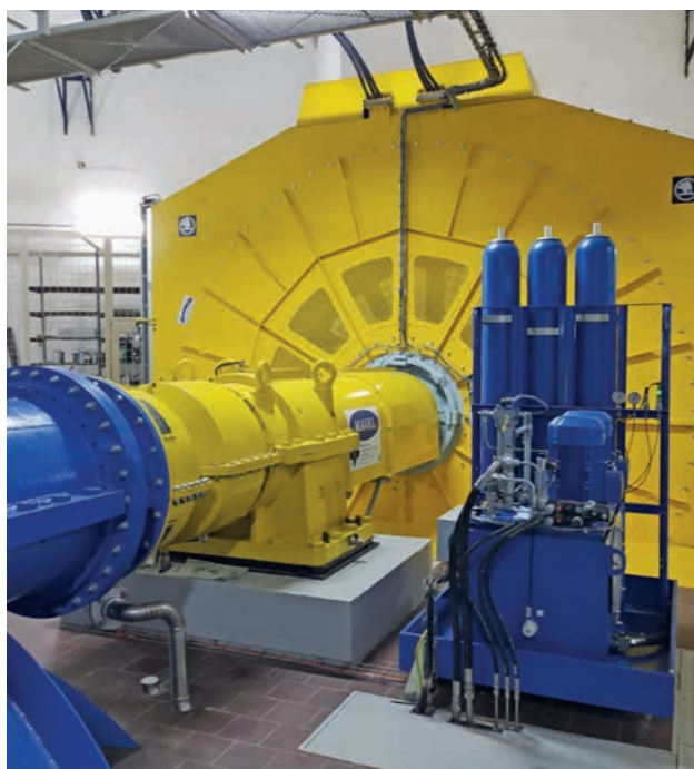
Small Hydropower Plant Štvanice (Author: Hubalová Petra)
