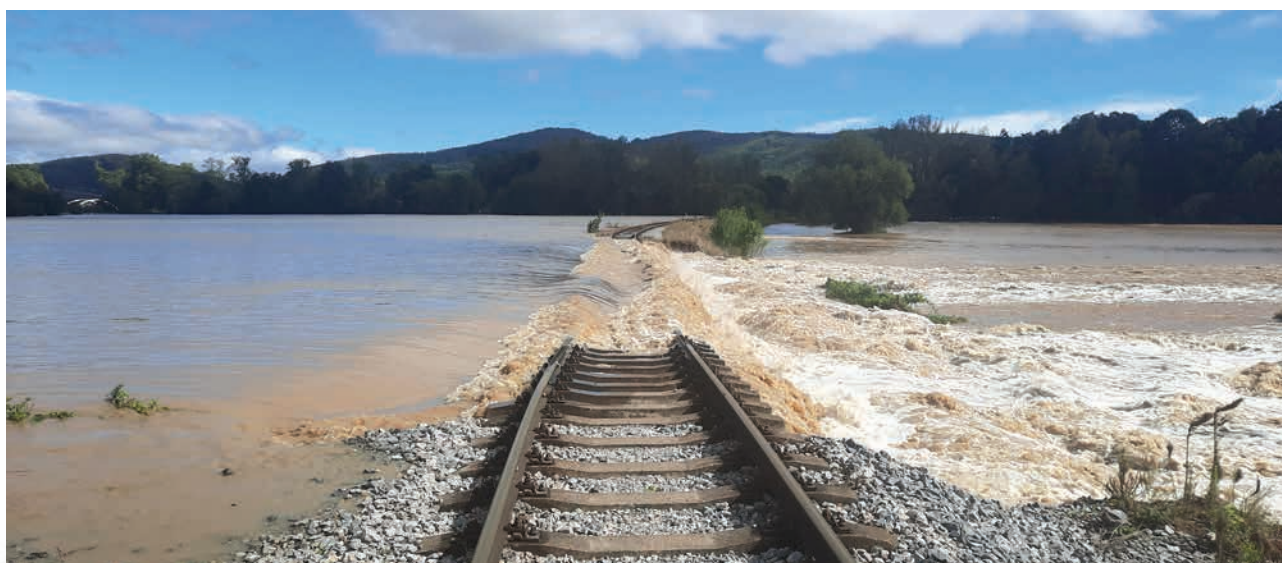
The Flooded Morava Stream damaged the railway tracks near the village of Leština (source: Morava River Board, s.e.)
