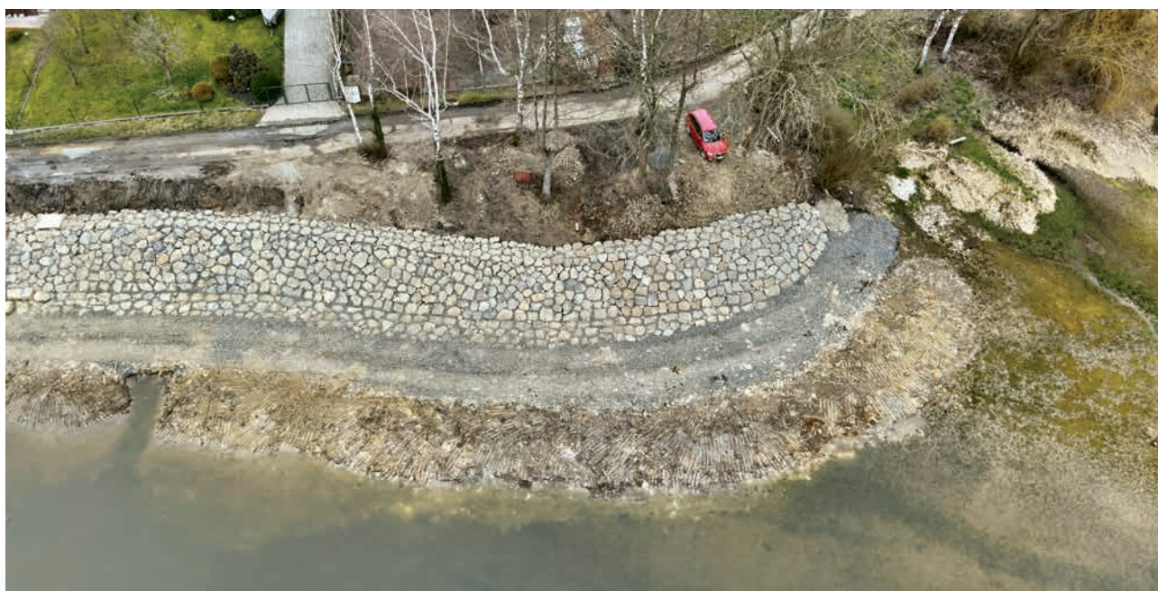
The Jesenice Reservoir, abrasion (source: Ohře River Board, s.e.)
