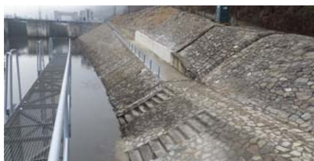
The Vltava River – Vrané – flood recovery (author: Hana Žáčková)
