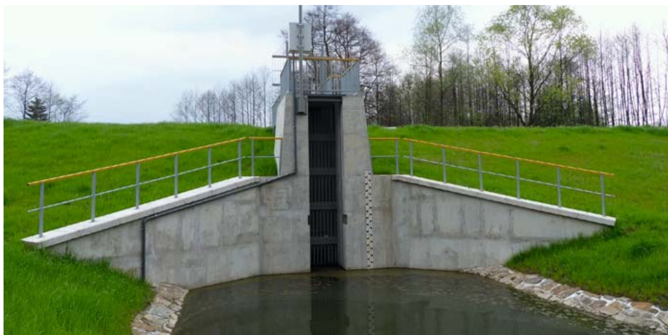
Dry reservoir Lutyňka (source: Oder River Board, s. e.)
