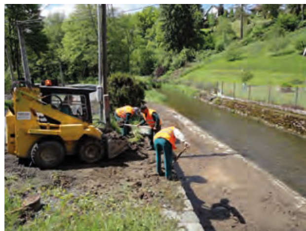
Operation and maintenance (source: Ohře River Board, s. e.)
