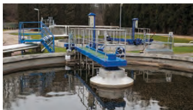
Pacov, intensification of a waste water treatment plant (author: Michal Němec)
