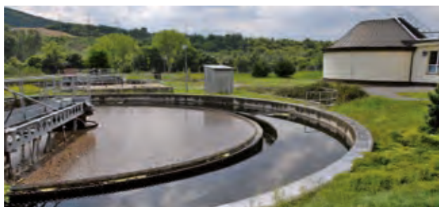
The waste water treatment plant in Beroun (author: Tomáš Petr)
