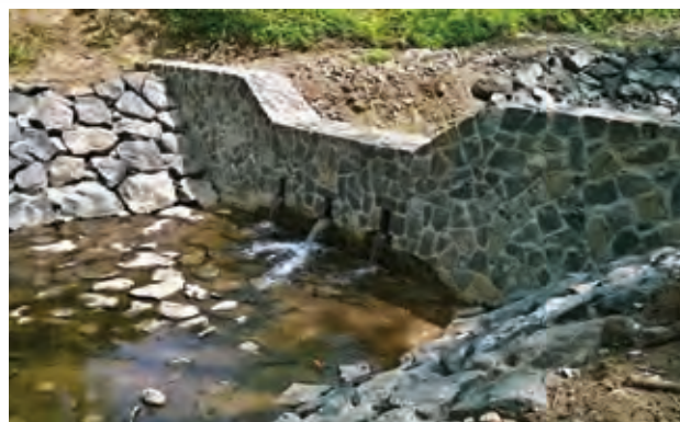
Regulation, Boletice (source: Ohře River Board, s. e.)
