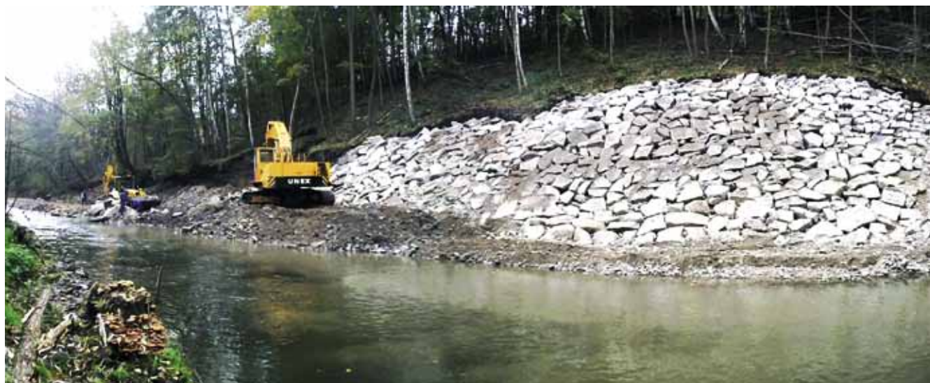
Flood control measures in the Lužická Nisa River in Machnín
