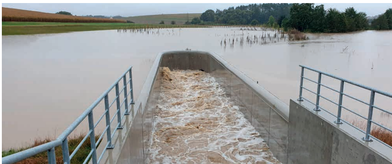
The Dry Retention Tank when capturing torrential rainfall, Mysločovice (source: State Land Office)
